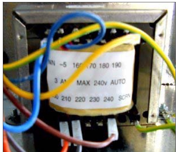
Fig. 5-12 Transformer - post November 2002
